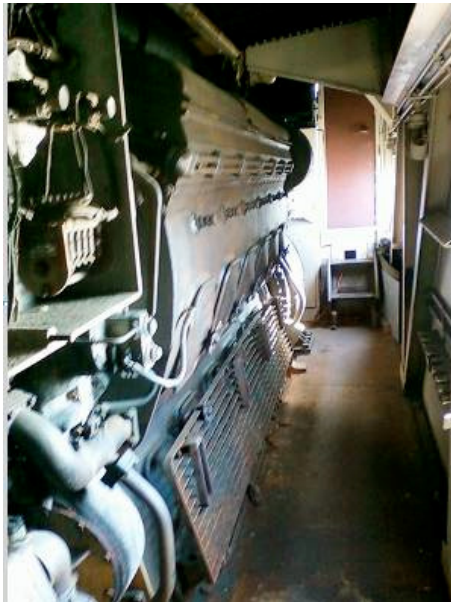
Above middle: Under the hood of an EMD locomotive – the long view.
